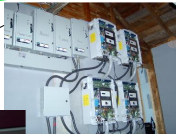
SunnyBoy ® with 2 strings of BP Solar Modules
