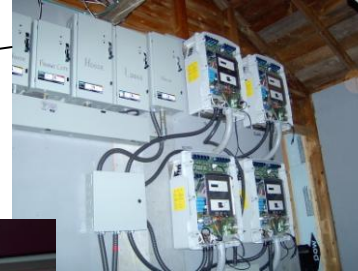
SunnyBoy ® with 2 strings of BP Solar Modules
