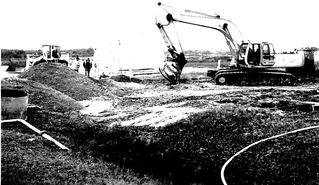
Photograph 4. Photograph facing north showing backfilling activities. Photo taken by Tetra Tech on August 28, 2013.
